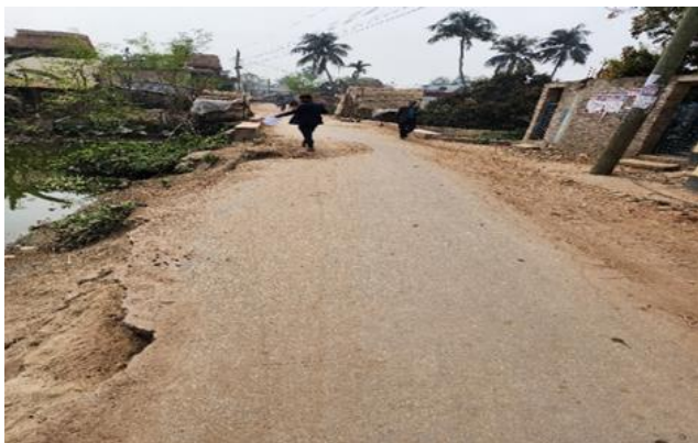
Fig. 8: Damage Road Surface Due to Lack of Maintenance (Road # 3)
