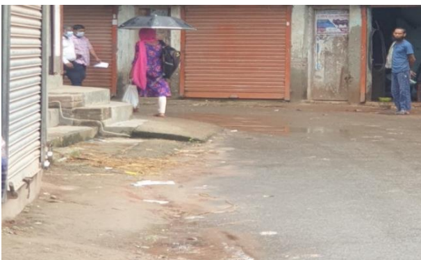
Fig.16: Roadside Open Drain Without Barriers (Road # 02)
