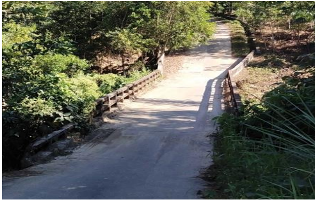
Fig. 21: Narrow Bridge Without Pedestrian Facilities (Road # 6)
